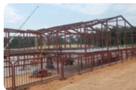
The Douglas County School System chose GreyStone Power over Georgia Power to supply energy to two new schools being built on Mason Creek Road.
